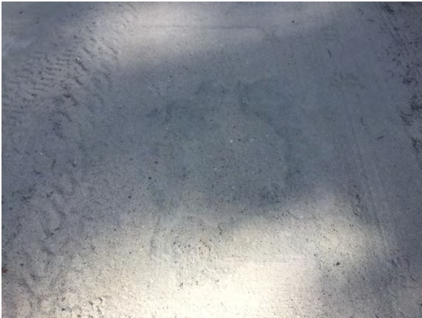
Appears as though grout was spilled on deck at some point
