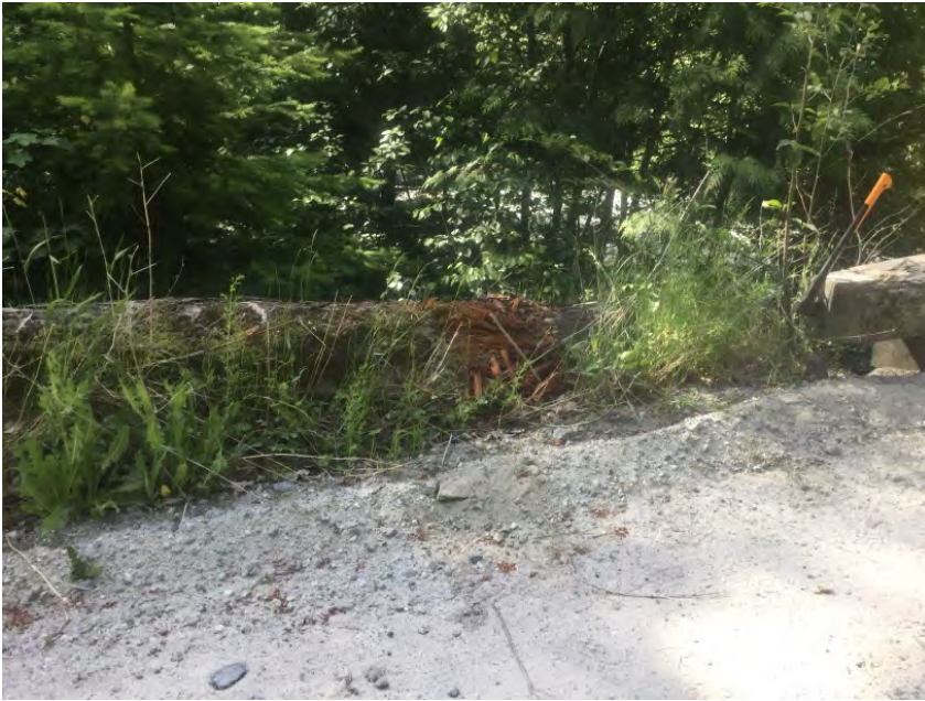
Rotten fender log downstream left approach
